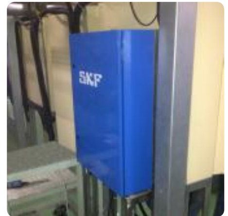
A NetEP cabinet in a permanent installation at a customer site
