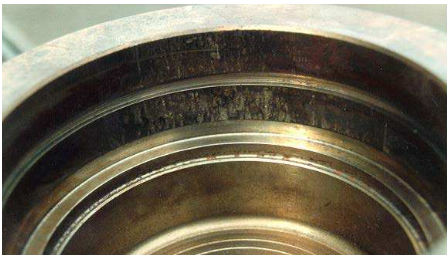
Fig. 7 Fretting corrosion in the housing
