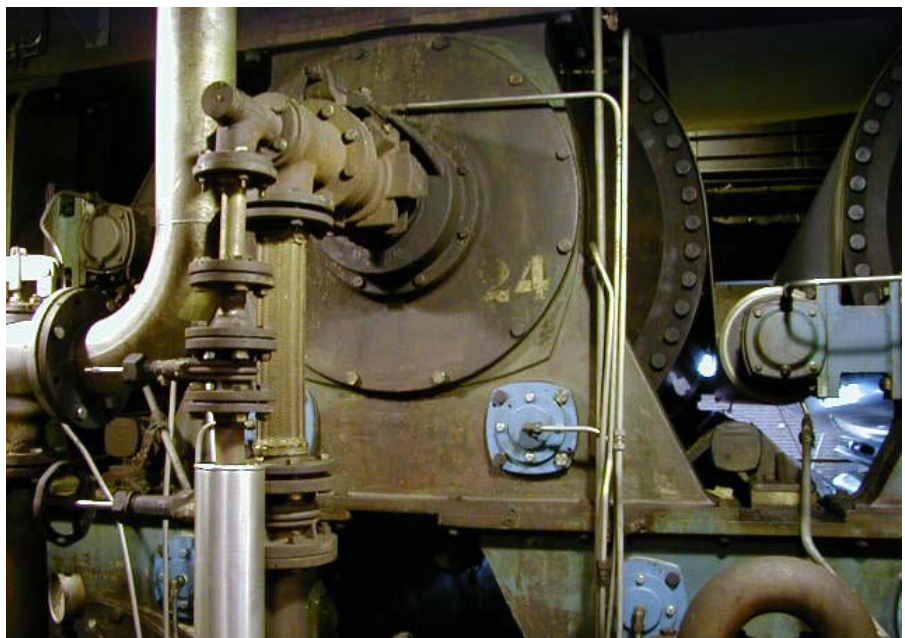
Fig. 5 Intermediate gears on a drying cylinder drive. Note that the blue covers show their position
