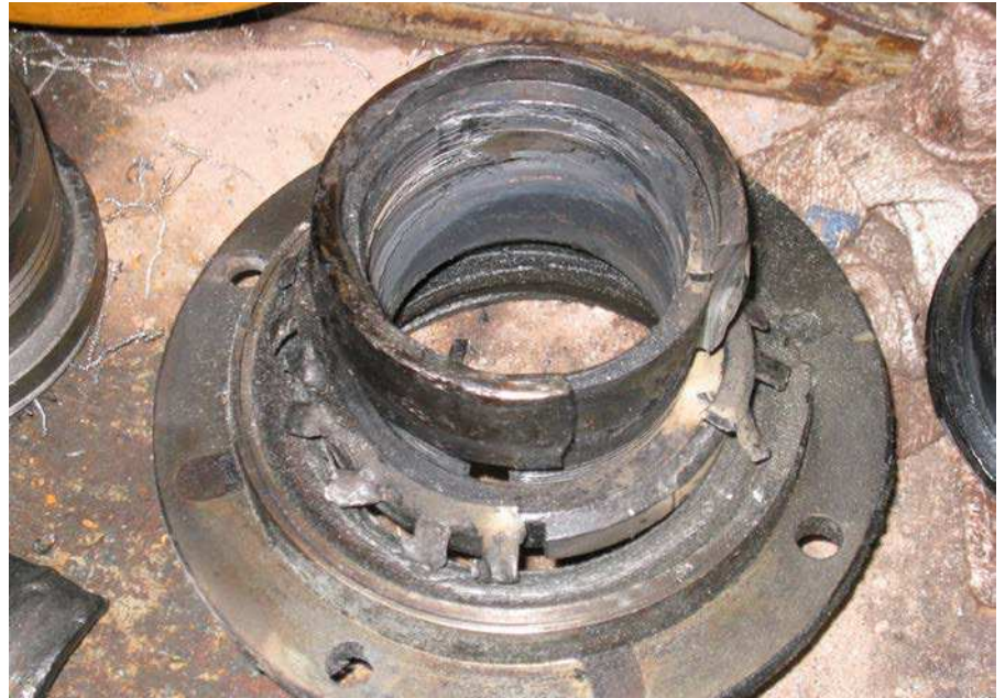
Fig. 11 Part of a bearing inner ring on an adapter sleeve following heavy damage
