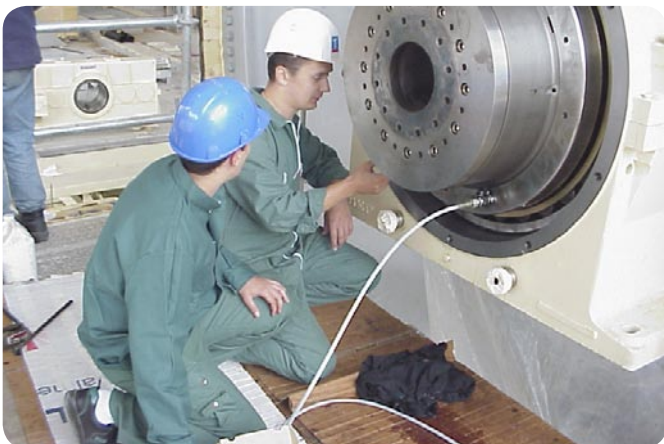
Fig. 8 A CARB toroidal roller bearing, mounted with the SKF Drive-up method, on a Yankee cylinder at Delipapier, France in 1999. The SKF engineer controls the axial bearing displacement indicated by the dial gauge that can be seen in fig. 9.
