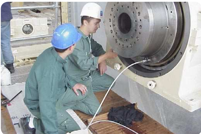
Fig. 8 A CARB toroidal roller bearing, mounted with the SKF Drive-up method, on a Yankee cylinder at Delipapier, France in 1999. The SKF engineer controls the axial bearing displacement indicated by the dial gauge that can be seen in fig. 9.
