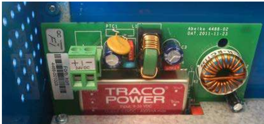
Figure 2 - 2. 24 V DC Power Supply Terminals.
