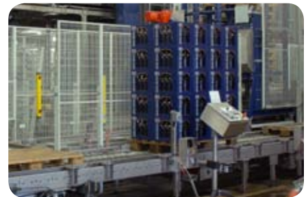
Palletizer with Lincoln lubrication system in a brewery
