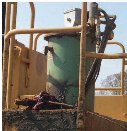
Example of reservoir overflowing that can cause slip-and-falls, fire hazards or other concerns.
