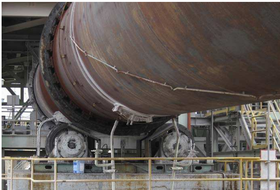
Fig. 3: Lime kiln support rollers
