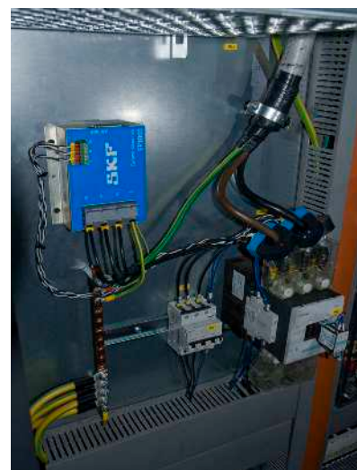
An EP1000 mounted inside a motor control cabinet with proper connections
