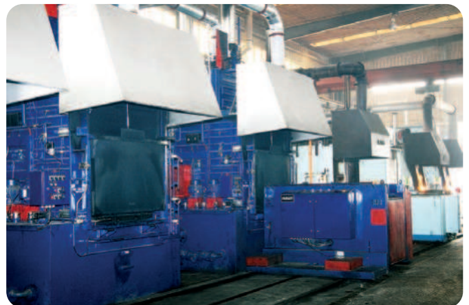
Furnaces for heat treatment process
